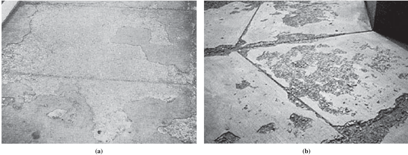
FIGURE 14 Concrete scaling (a) and spalling (b) [adapted from Potomac Construction Industries (2007) and Cryotech Deicing Technology (2007), respectively].
