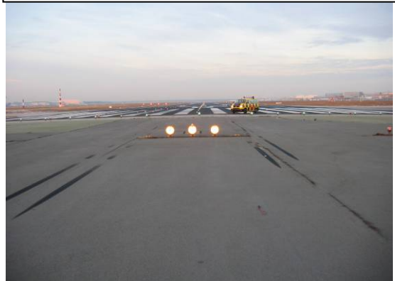
Touchdown marks and two missing approach lights (right and left)
